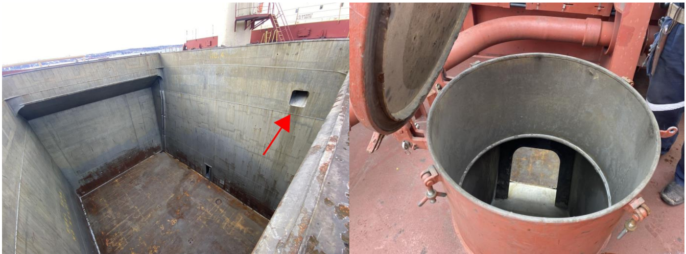
Figure 7-16: Manhole for Baghouse Ductwork Connection
